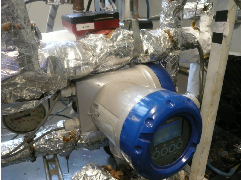
Figure 34. Overall View of the Flow Meter
