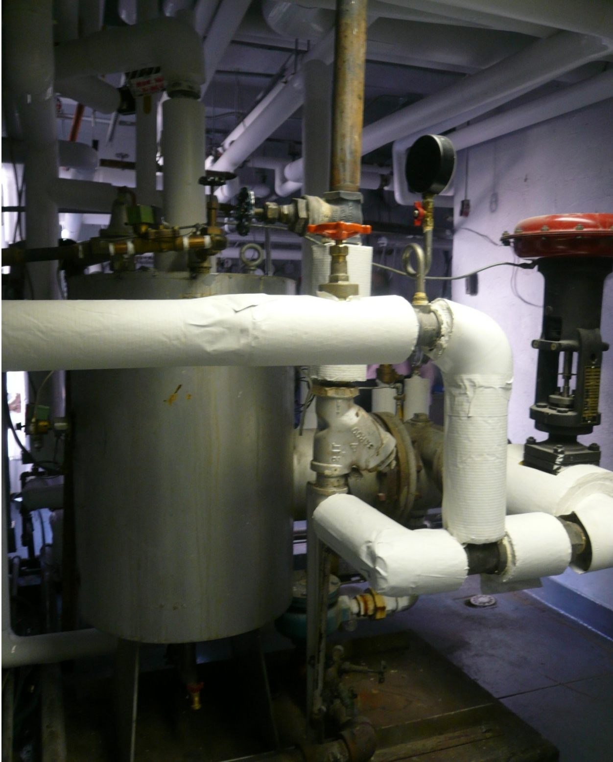
Figure 36. Rear View of Existing Patterson Kelly 400 Domestic Hot Water Unit
