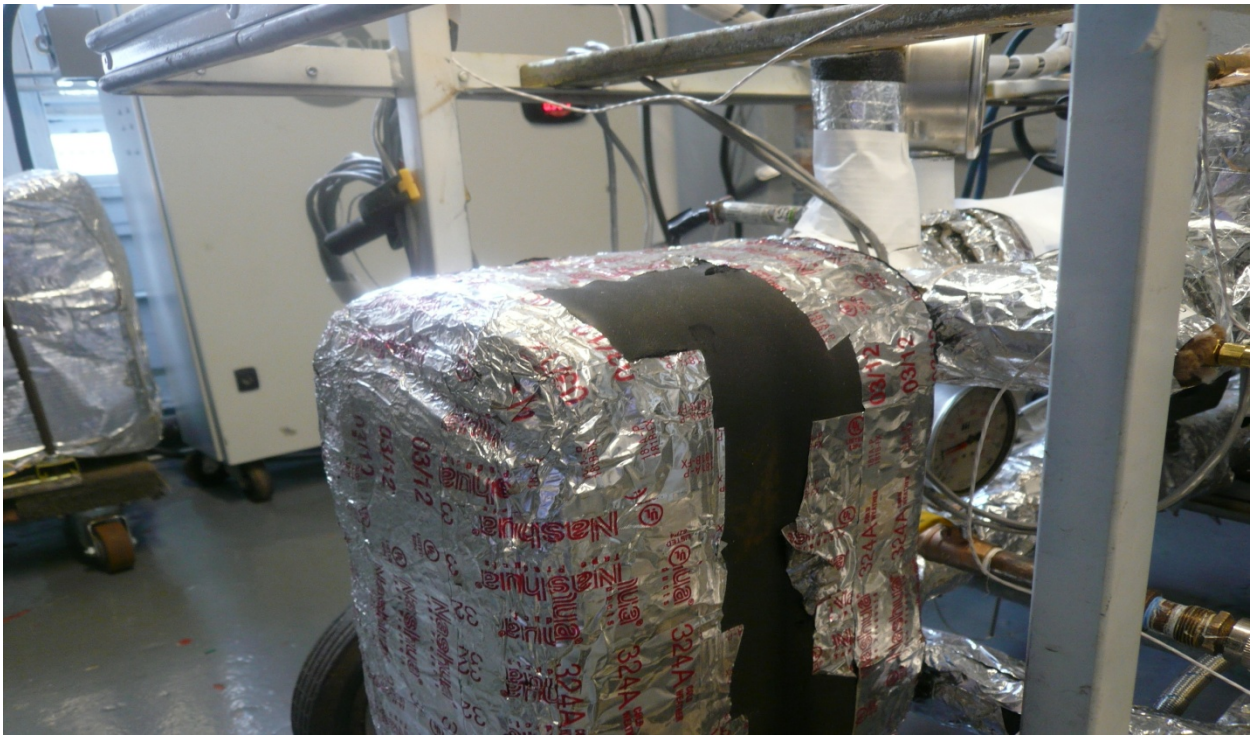
Figure 30. The Main Heat Exchanger (HX1)
