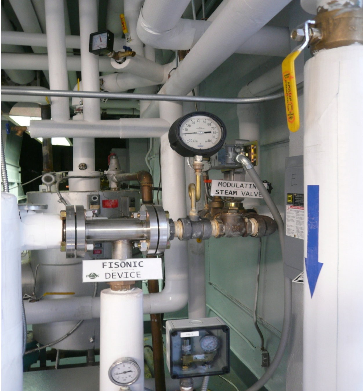
Figure 41. The Fisonic Device and the Modulating Steam Valve of the New Unit
