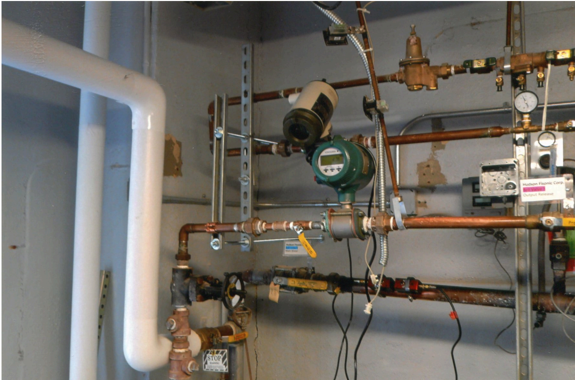
Figure 14. Cold and Hot Water Flow Meters
