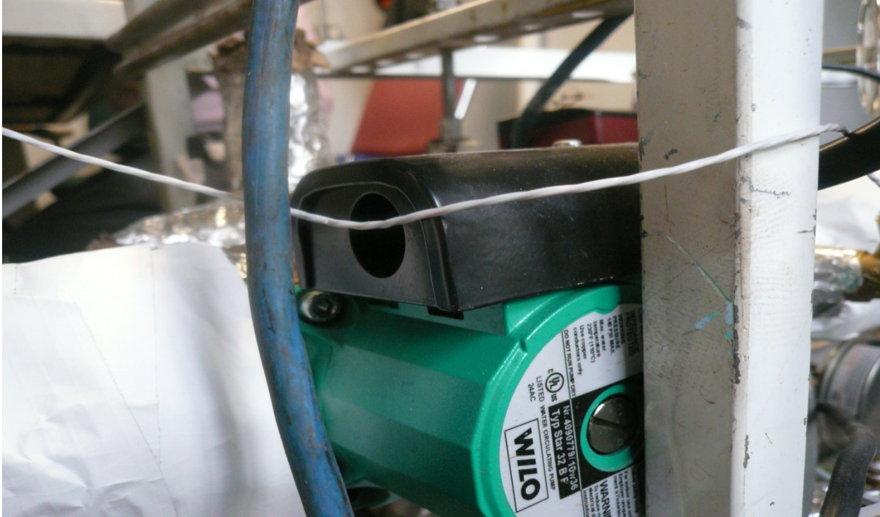
Figure 31. The Primary Loop Water Circulating Pump P-1 (Wilo)
